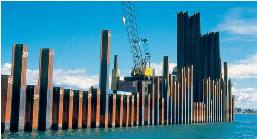
The project's design lifetime of 50 years called for two layers of tar-free epoxy coating
